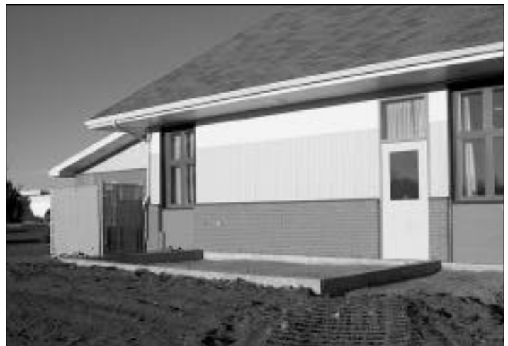
Much needed storage space was added onto the Blackburn Community Hall in November. This was jointly funded by the City of Ottawa, Recreation and Parks Board (RPB) Reserves, RPB Minor Capital, Community Hall revenue from 1998 - 2000 and the Blackburn Community Association.
